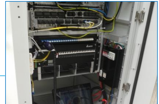
BBU and Fiber Patch Panel
